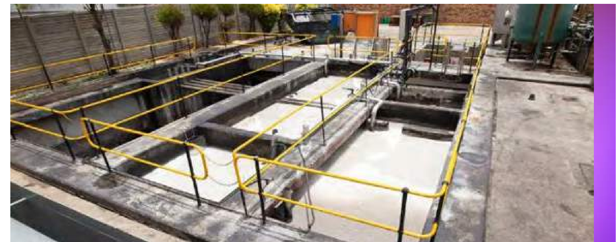
Figure 24: Effluent treatment at Tanker transport facility in Germiston
